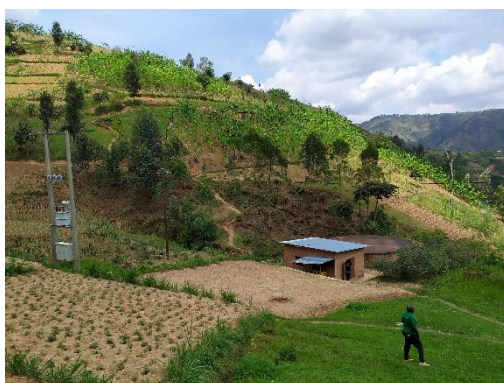
Station de pompage Munyana – Station de pompage
